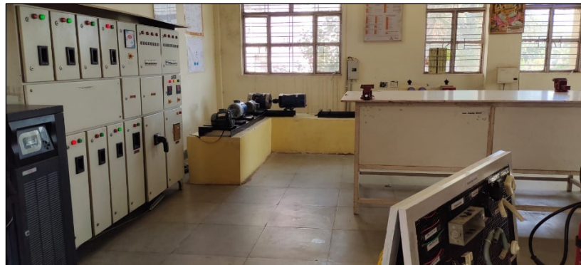
Figure 8 : Infrastructure & equipment provided by GAIL
